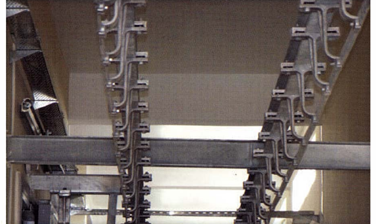
CORIDOR MONORAIL LINE
