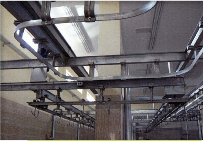
SHEEP BLEEDING AND CONVEYOR
