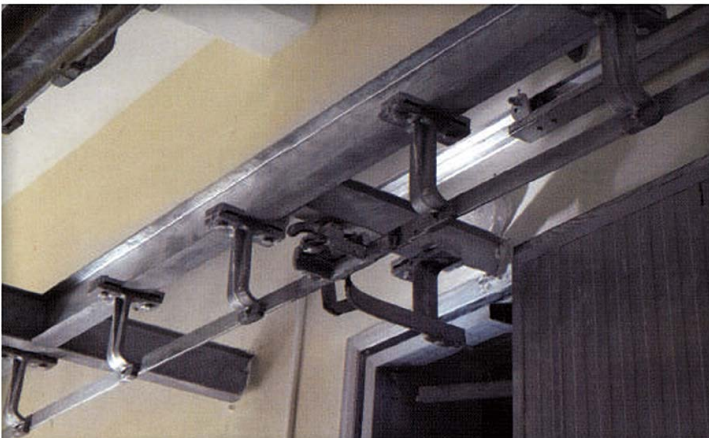
COLD STORAGE INLET
